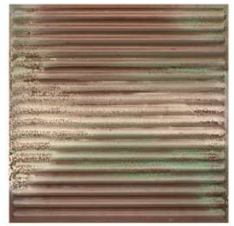
261 - Corroded Metal (V1)
